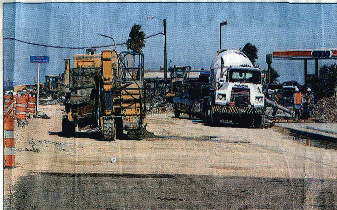
Crews work on Ennis Joslin Road. Some local American Indians are angry that the state highway department has contracted out construction on the road for years, aware that it runs over an ancient Indian burial ground. The highway department says Indians were consulted in the planning stages.
